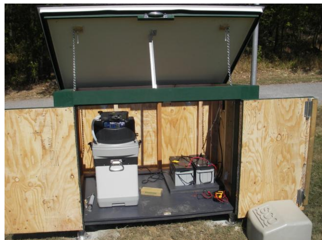
Automated stormwater sampling system.
