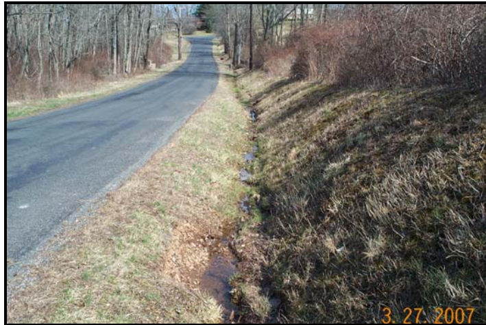
SDO-13&15 Ditch with steep side slope
