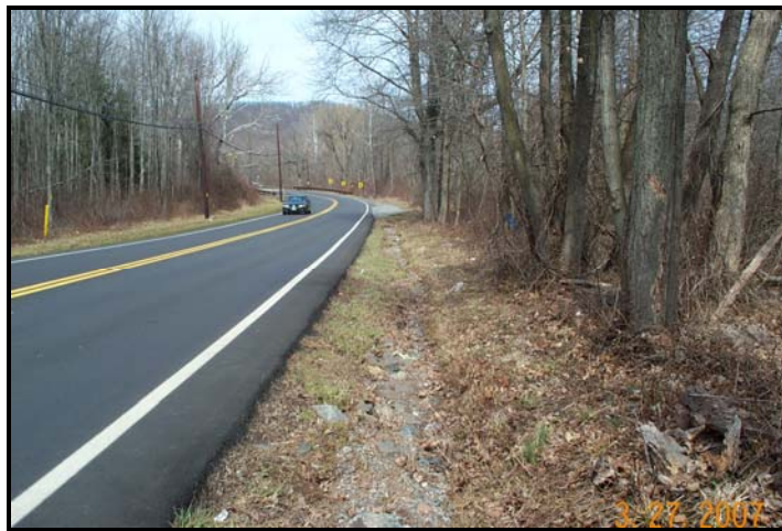
SDO-186 Ditch with sediment deposition in channel
