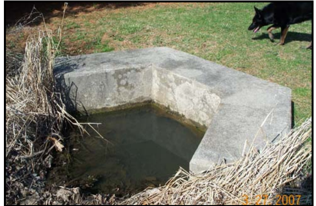
Stormwater discharge filled in with debris
